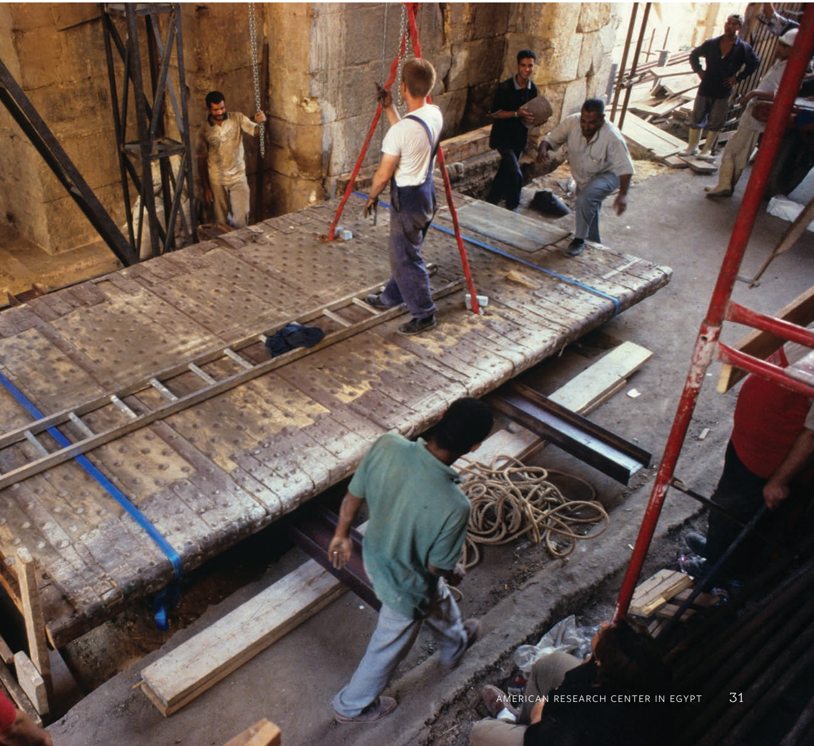
Cutting the foot of the east door of Bab Zuwayla before its removal for restoration
