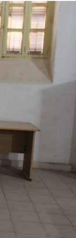
LEFT: Carter’s study, pictured as it was during initial assessments of the house in 2020. The space was previously used as a screening room that featured a now-defunct hologram of an actor speaking as Howard Carter. PHOTO: SALLY EL SABBAHY
